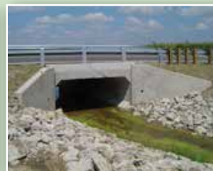
Highway Crossing Drainage
